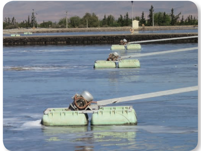
OxyStar ® Aerators in Operation
