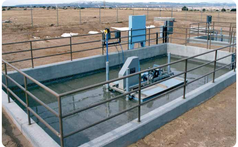
Overview of the AquaCAM-D® unit in a SBR reactor.
