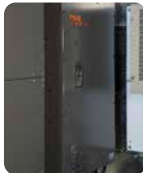
PWM Power = Lowest Harmonics
