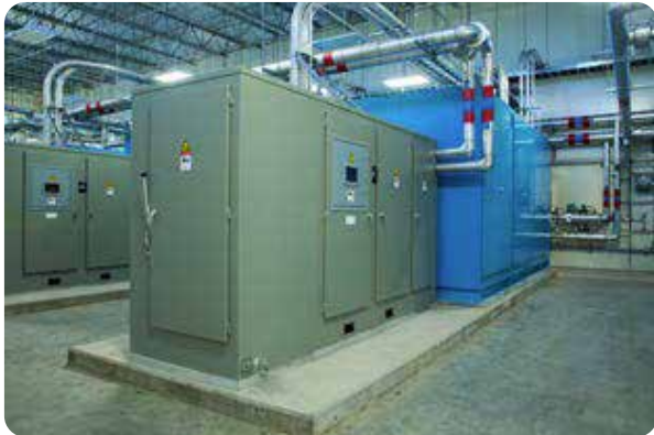
Power Supply Units
