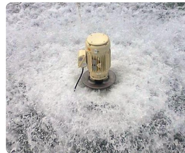
Aqua-Jet® aerator model SS-PW in operation in a TTHM stripping application.
