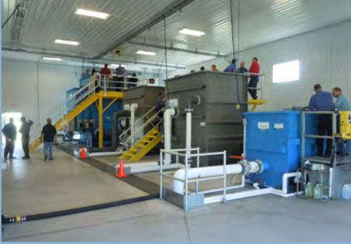
Aqua-Aerobic Research & Technology Center
