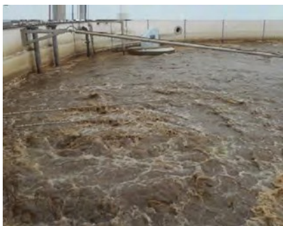
Compromised Aeration Piping of Fine Bubble Diffuser System
