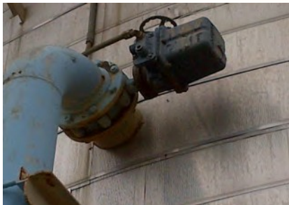
Valve Actuator Issues
