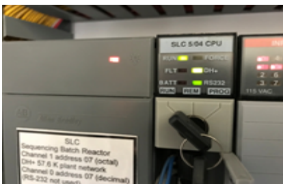
Obsolete Allen Bradley PLC
